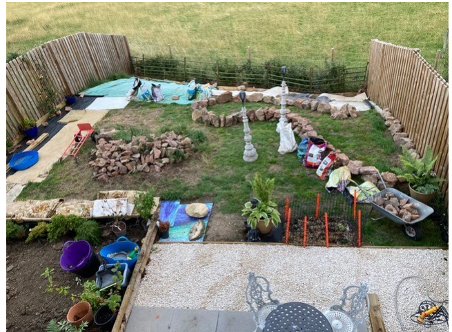
Plan for paths, raised beds, seating and planting completed so construction in progress ....
